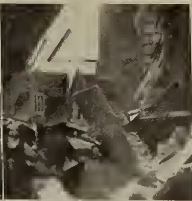
2. HOLE IN GREEN HALL ROOF.
